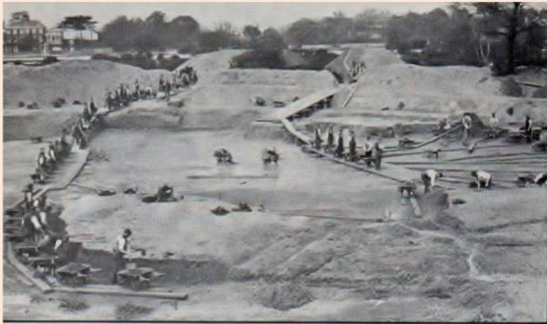
Excavations by hand for Whipps Cross Lido in 1907 as a winter unemployment relief scheme.
